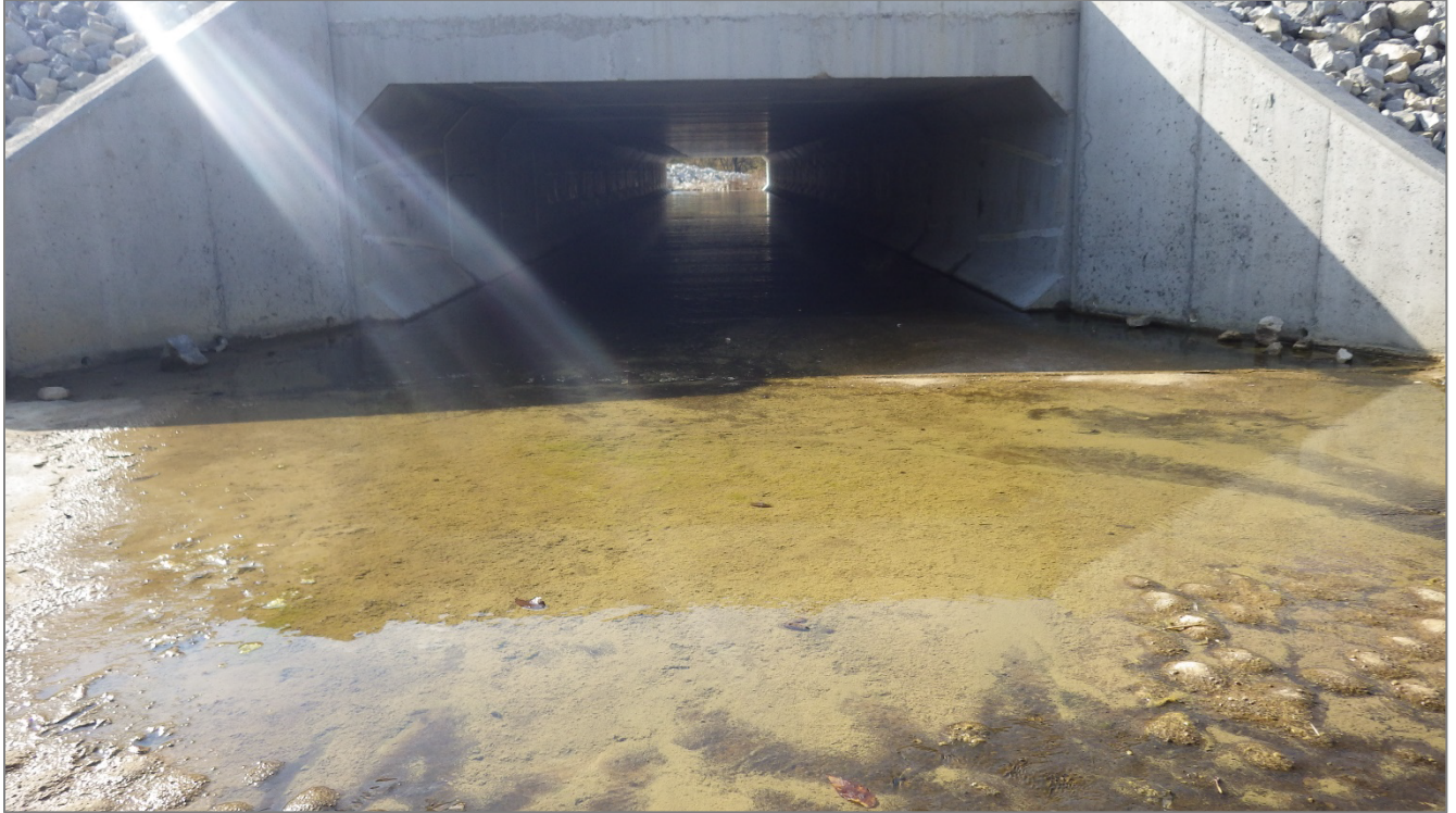
Photograph 11 – Upstream side of dam at 12 ft. x 4 ft. culvert, looking southwest through the culvert.
