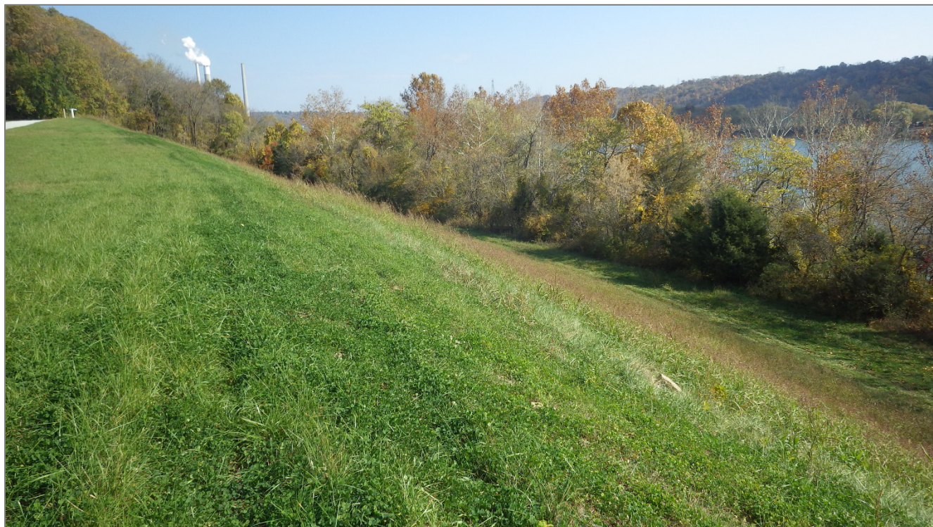
Photograph 9 – Crest of dam near center, looking east. Note tall grass on downstream slope.
