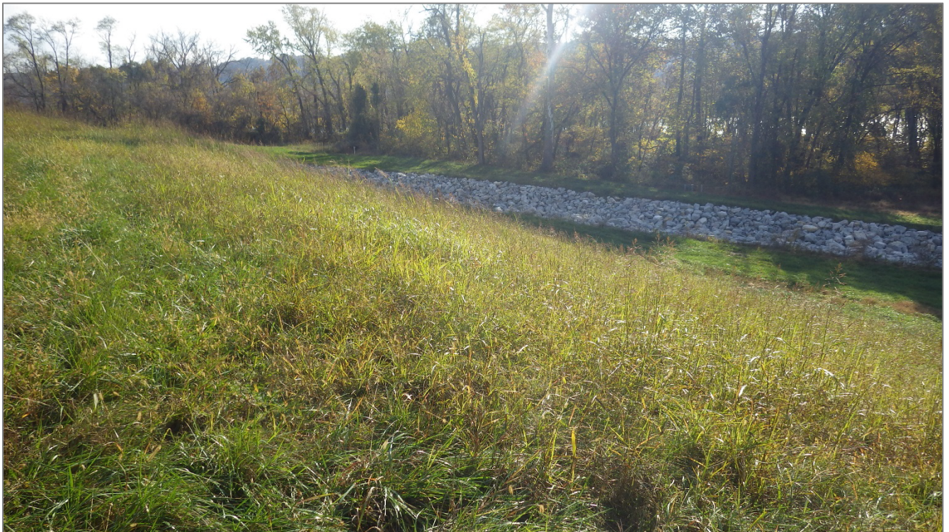
Photograph 6 – Western downstream side where the channel extends along the face and toe of the embankment. Note tall grass along slope.
