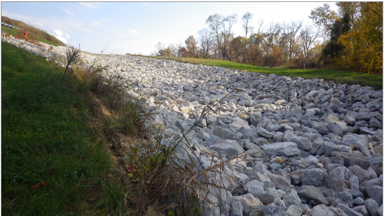
Photograph 4 – Western downstream channel showing erosion due to material change and silt fence removal.
